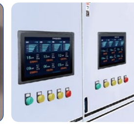
Power grid control cabinet
